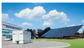
Trend-setting: The “cellcube” large battery is used at the Bielefeld site for lighting the factory premises and as a planned solar service station.
